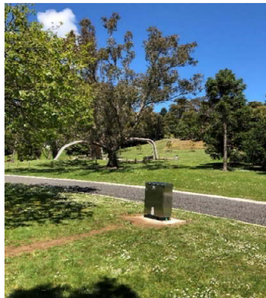
Figure 19: Power outlet at roadside
